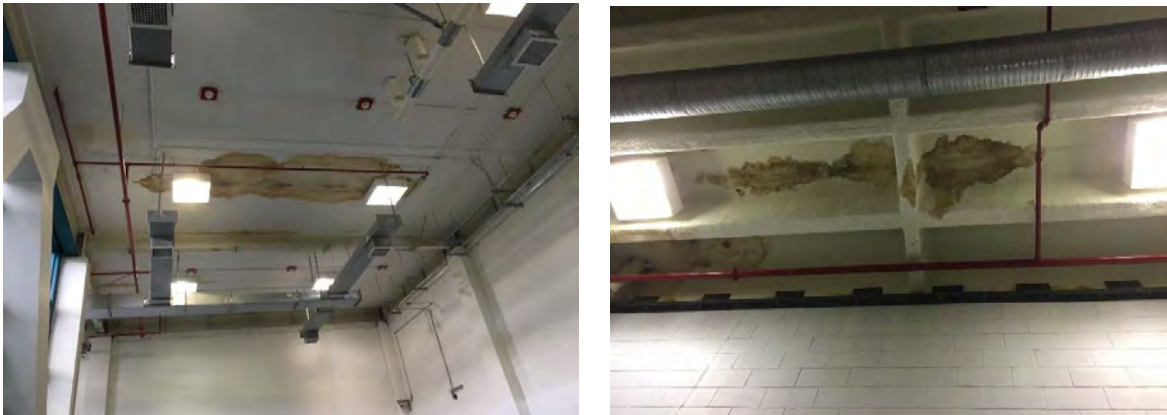
Figure 4. Roof leaks found in every housing unit. Observed by OIG at the Essex Facility on July 24, 2018. Source: OIG
