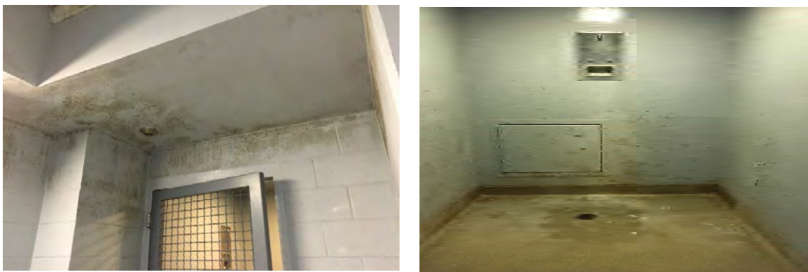
Figure 5. Hallway leading to shower filled with mold and shower stall with mold, mildew, and peeling paint. Observed by OIG at the Essex Facility on July 24, 2018. Source: OIG
