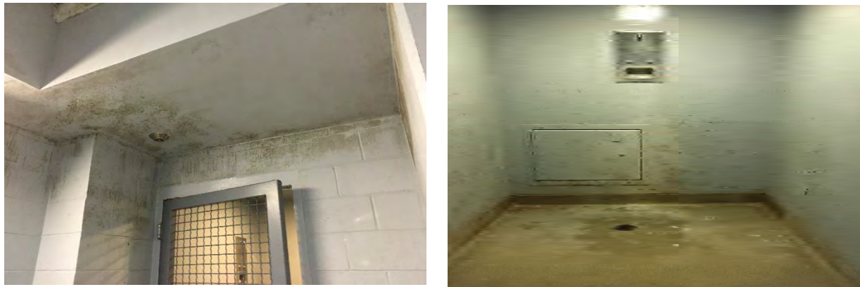
Figure 5. Hallway leading to shower filled with mold and shower stall with mold, mildew, and peeling paint. Observed by OIG at the Essex Facility on July 24, 2018. Source: OIG
